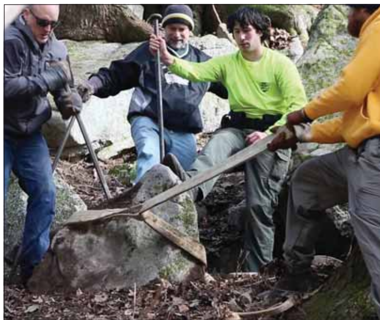
Volunteers work together to assist South Cumberland Park Ranger Park Greer (second from right) in excavating a large rock for use in a new rock staircase along the Fiery Gizzard reroute. Photo by Rick Dreves
